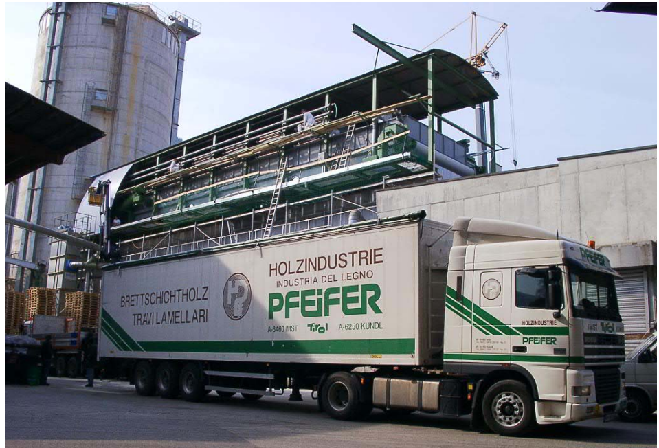
Figure 1 The 2 nd KUVU belt dryer at the premises of the company Pfeifer in Kundl, installed above the first dryer, right before completion
